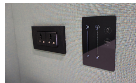
LED Screen with Adjustable Ventilation & Lighting controls
